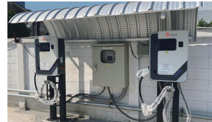
SCB charging station
