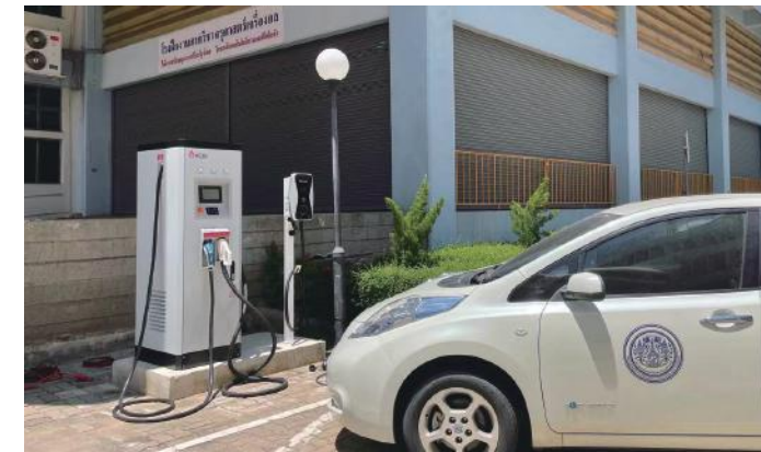
KMUTT University charging station
