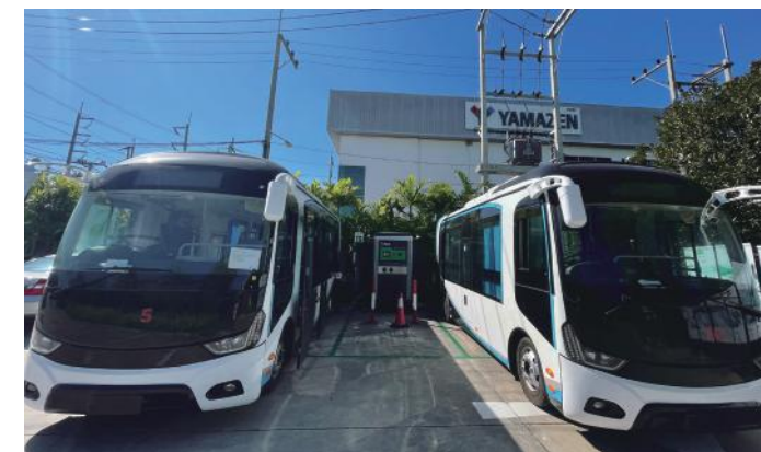
Bus charging station
