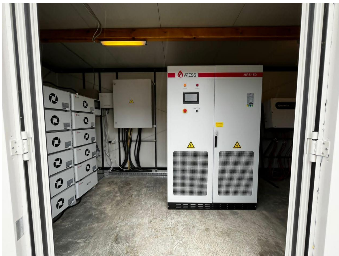
ATESS HPS150+BR157 battery bank installed for a glass factory in Romania to reduce energy cost
