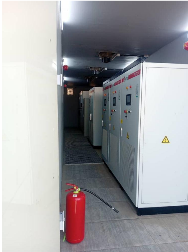
Two ATESS PCS500 battery inverters
