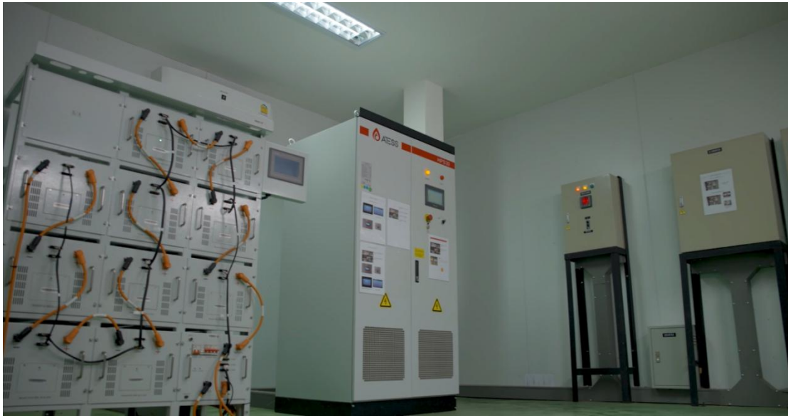
The HPS30 and battery systems installed in the Banmai Hospital
