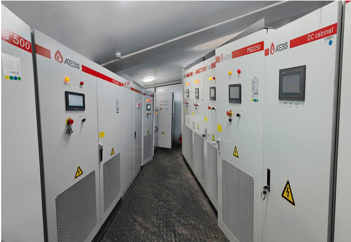
2 sets of ATESS PCS500 battery inverters and other components installed for the Saudi Arabia Project
