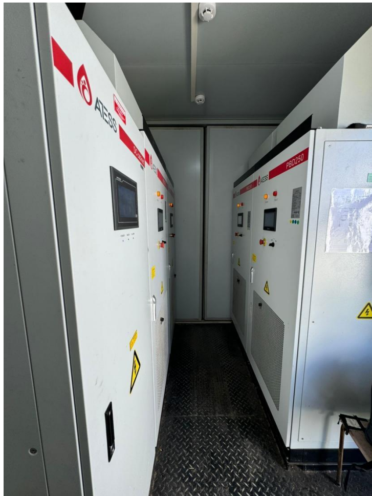
ATESS PCS500 energy storage system installed for RFM project
