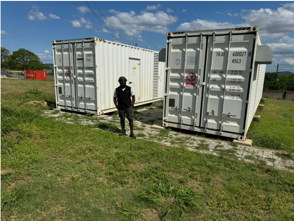
ATESS South Africa After-sales Technical Support Engineer stands around this project’s BESS Containers
