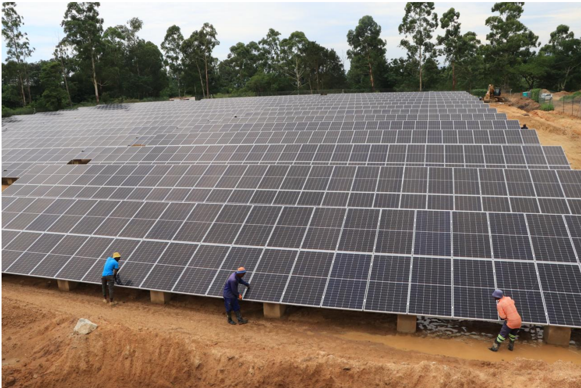
The onsite 1 MW PV Array at Raleigh Fitkin Memorial Hospital (RFM) Project (Image source: www.undp.org )
