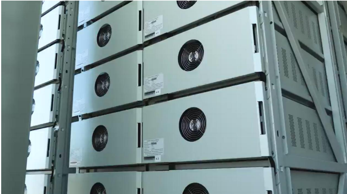
2.5 MWh ATESS battery system
