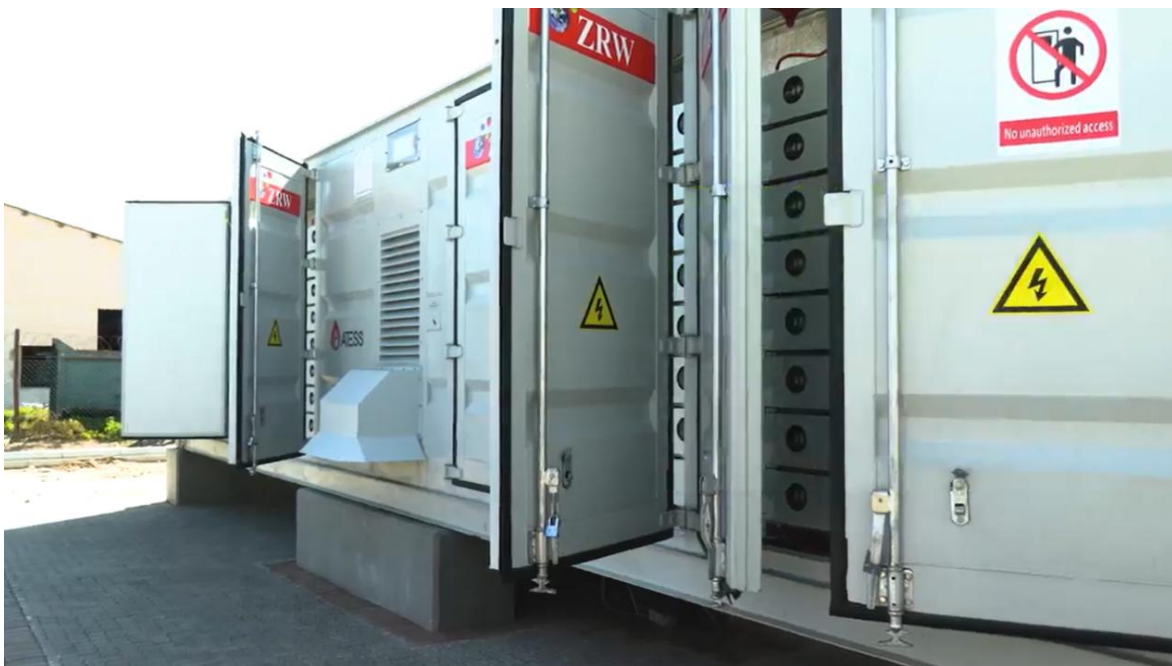
2 sets of ATESS 40HC BESS Container
