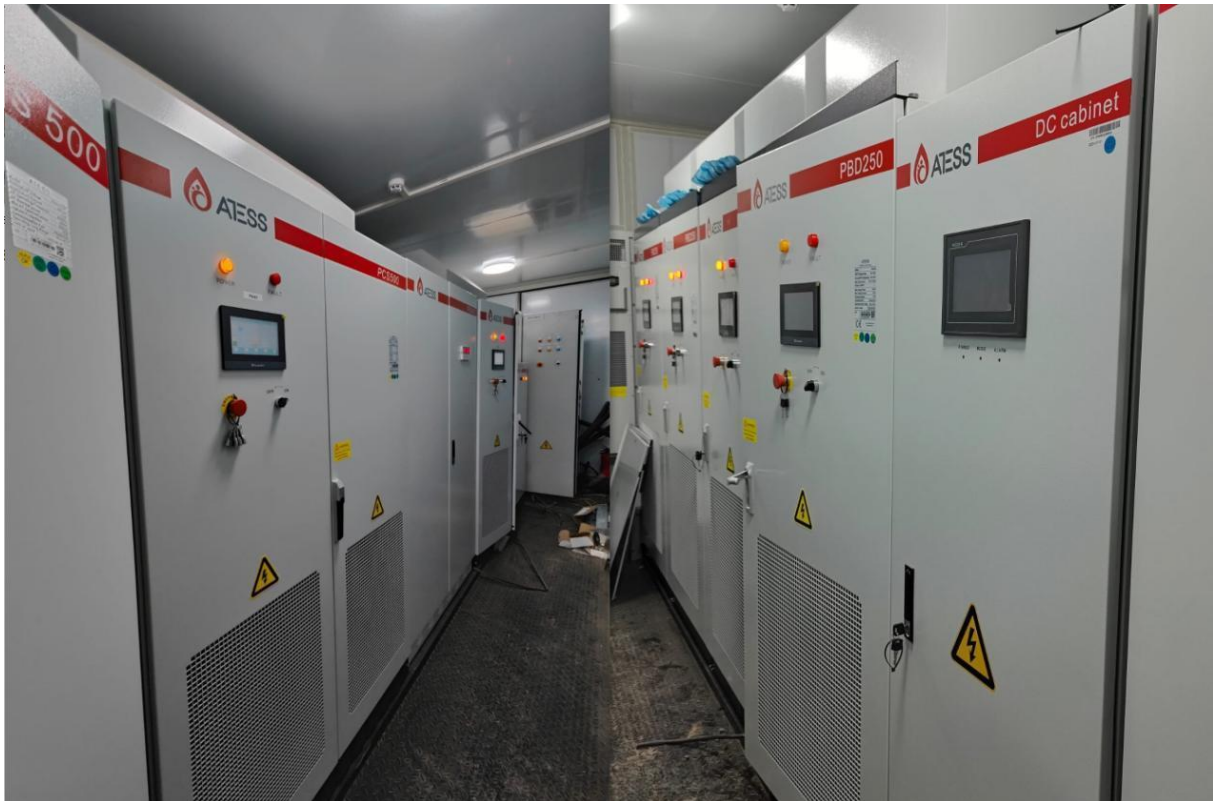
2 sets of ATESS PCS500 battery inverters and other components installed for the Saudi Arabia Project
