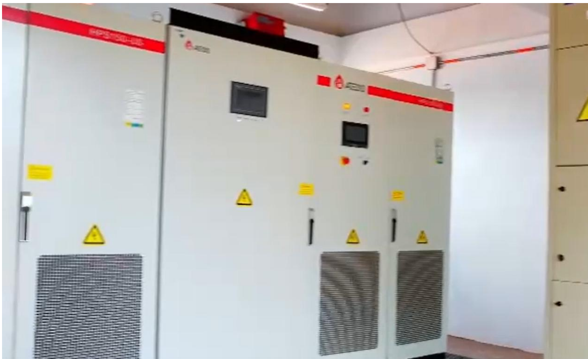
Two sets of 150kW ATESS HPS hybrid inverters
