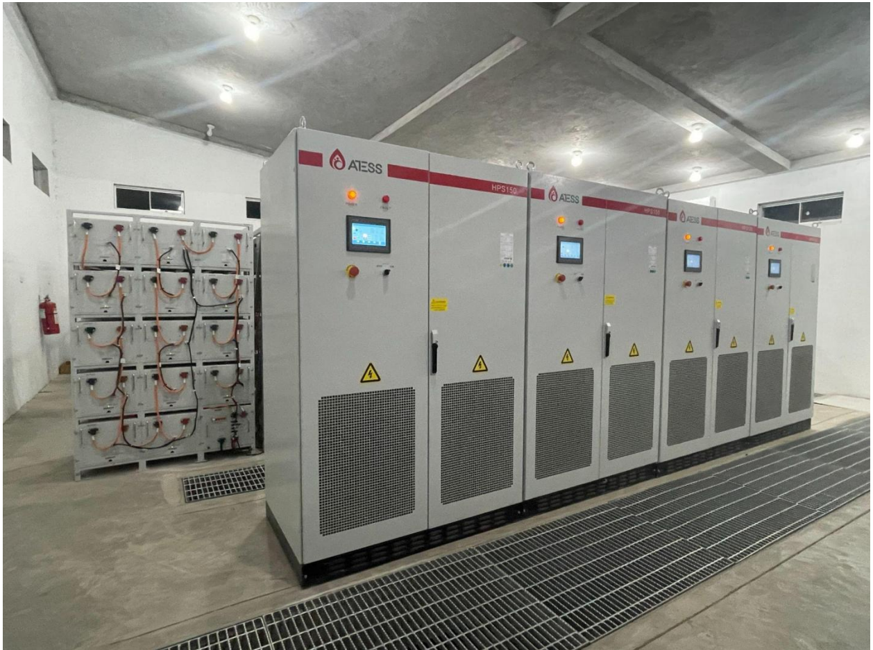
540 kW, 1,666 kWh ATESS Battery Energy Storage System (BESS) in Bretaña, Peru
