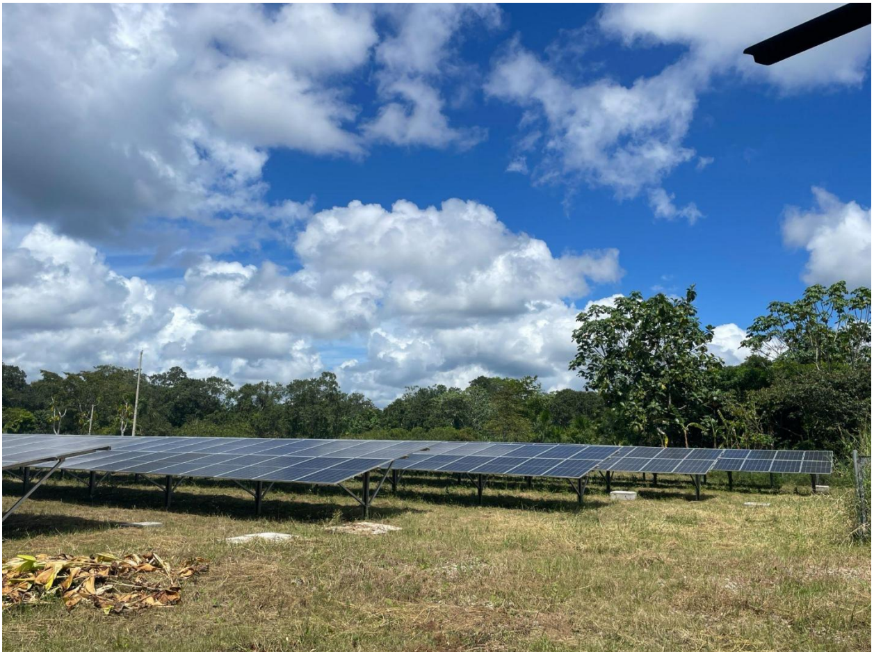
The installed PV system integrated with ATESS Battery Energy Storage System (BESS) in Bretaña
